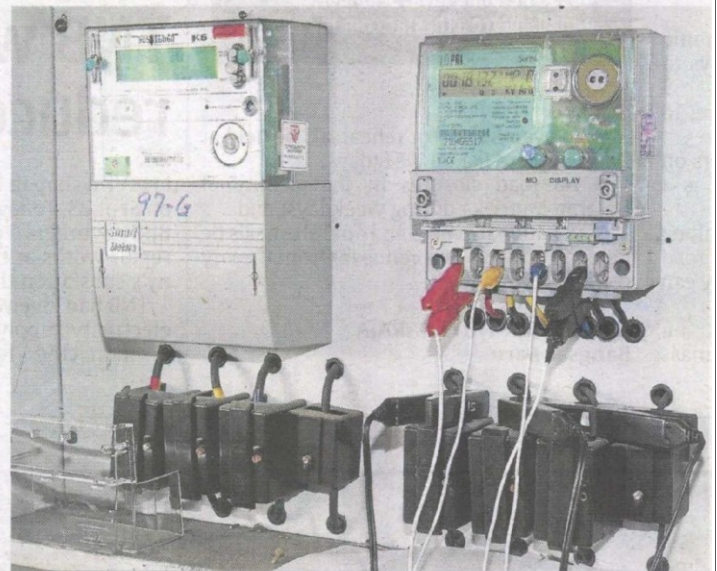
Commercial vs residential: A three-phase electricity meter is commonly used for commercial premises.
