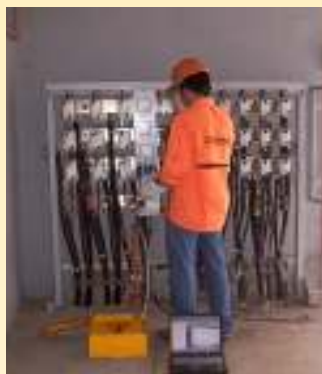
RESMOS Installation on Low Voltage Board
